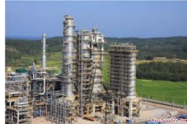
Nhon Hoi Refinery
